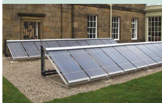
Solar thermal panels at Denton Hall © NG Bailey
